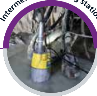
Water Recovery / Intake
